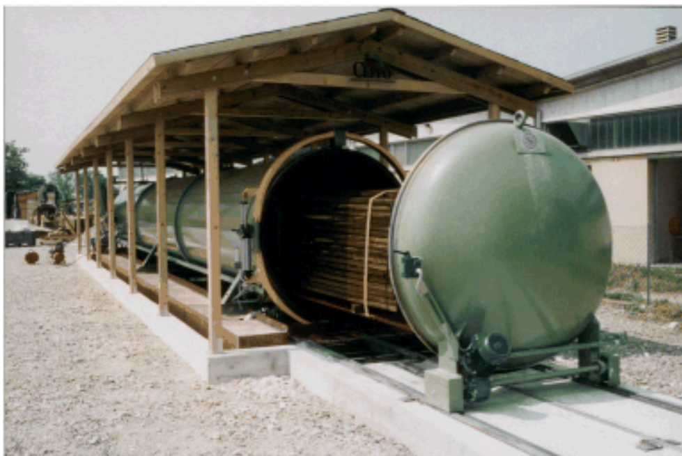
IMP-Vp plant installed at the company "Il Ceppo"
